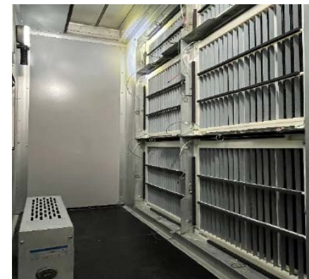
Air handling units installed at YG new office building where the filter is installed
